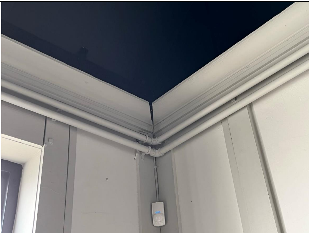
Photo 6 Opening of timber finishes attached to bowing wall, with electric cable in gap
