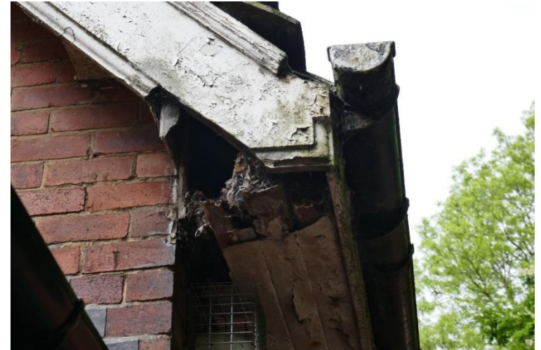
Photo of rear rainwater gutter and roof fascia / soffit detail showing major deterioration in timber panelling, due to missing and cracked roof tiles. Also showing evidence of bird nesting.
