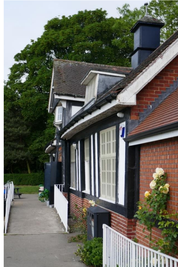
Photo looking west along the south facing front elevation showing the bowing out and leaning in the front wall and roof line to the front façade. Also note the dormers leaning back into the snagging roof line.
