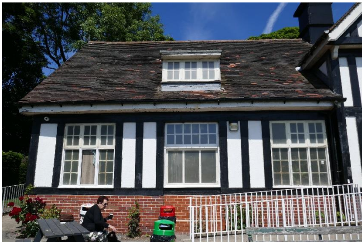
Photo of front elevation tiled roof finish showing missing and cracked roof tiles. Also note broken and boarded-up windows and blocked up clock tower.
