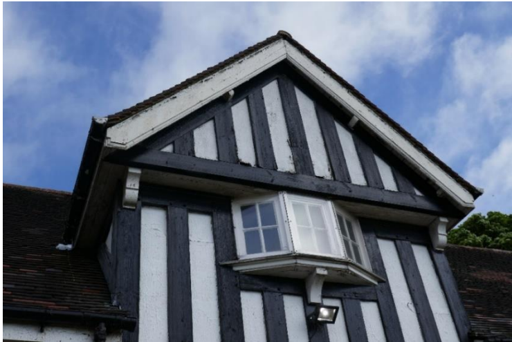
Photo of front elevation gable showing holes in the timber and render panelling, and the deterioration of the roof fascia, soffit and underside of window over main entrance.
