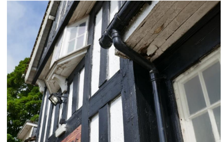
Photo of front elevation gable and roof fascia / soffit showing deterioration in timber soffit and bowing in timber panelling.
