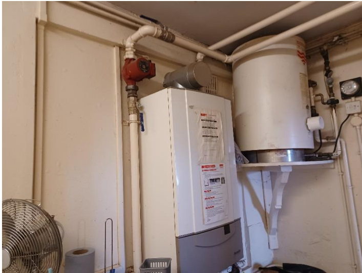
Photo showing existing boiler and hot water storage system.
