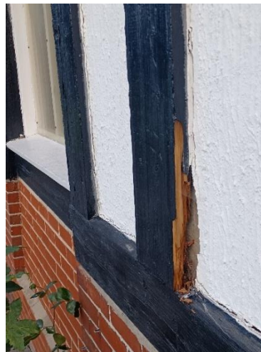
Photo of front elevation showing deterioration and cracking in timber and render façade.
