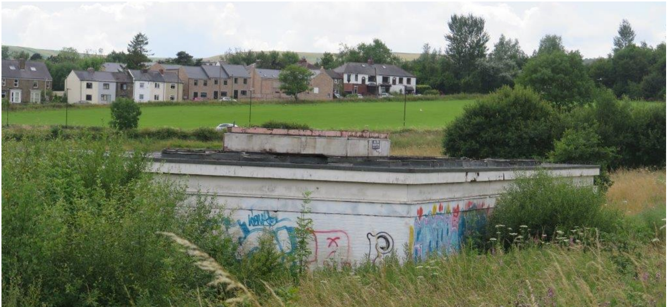
Derelict Sports Pavilion off Cross Lane
